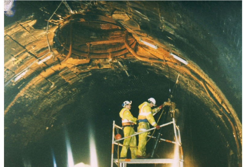
«Beacon Hill Tunnel, Halifax». Rock bolting next to tunnel ventilation shaft eye in 1995. Andrew Boggett.
