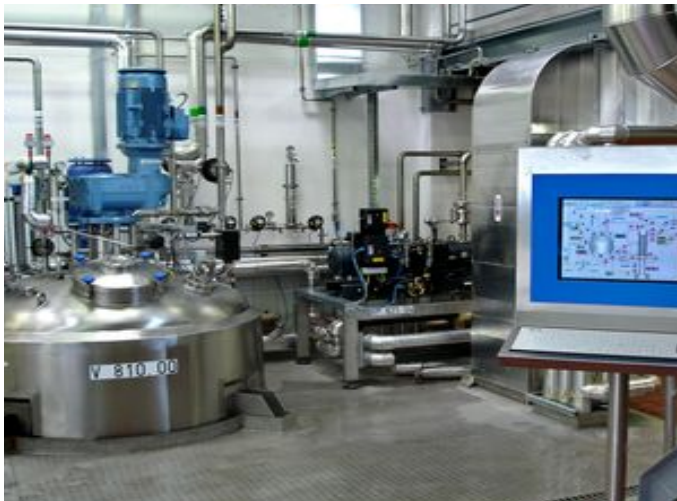
Recipe management system Batch in a pharmaceutical company to produce generics. http://www.kolektorautomation.com/index.php?t=referenceNews&l=en&id=60 .
